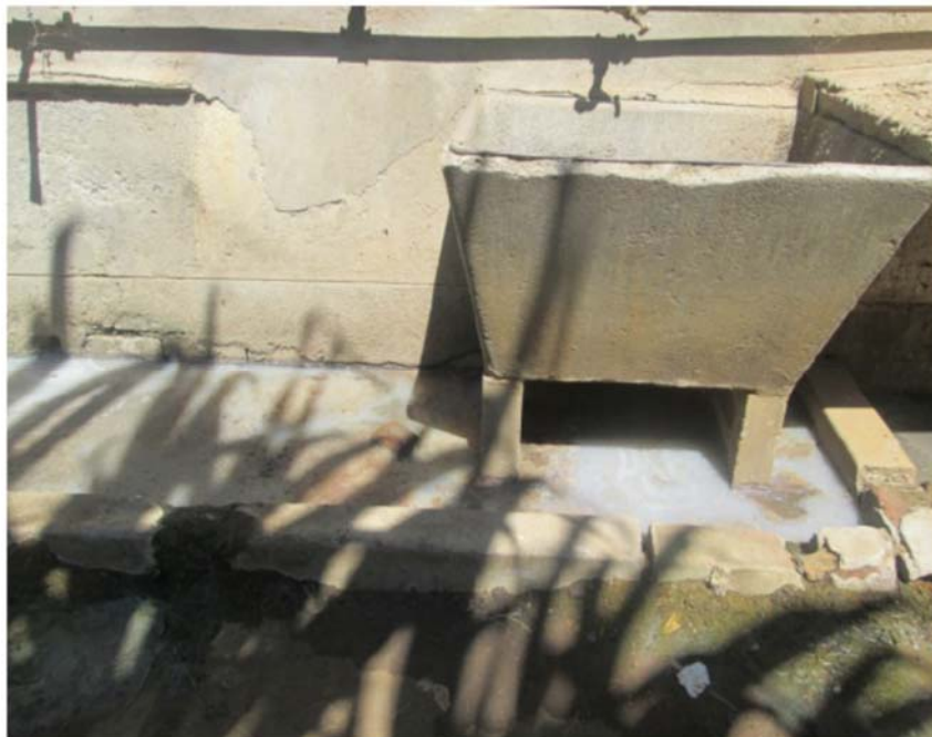
Plate 1. Blocked Sewer behind a communal toilet at the Uniformed Forces Compound
